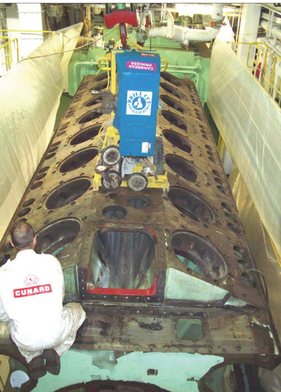
Fig 1 The engine to be removed weighed 58 tonnes and was 7500 mm long x 2450 mm wide and 2350 mm high
